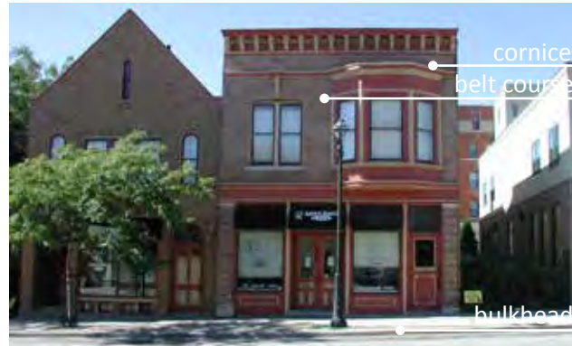
Fig B.2.C.4 INSIDE THE TRIANGLE: Horizontal elements, including a series of belt courses, the cornice and the bulkhead, establish rhythm in the storefront.
