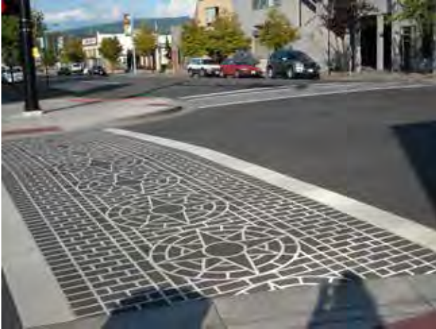
Fig. A.2.D.4: Bump-outs and crosswalks with decorative paving are present on primary internal drives when parking is included.
