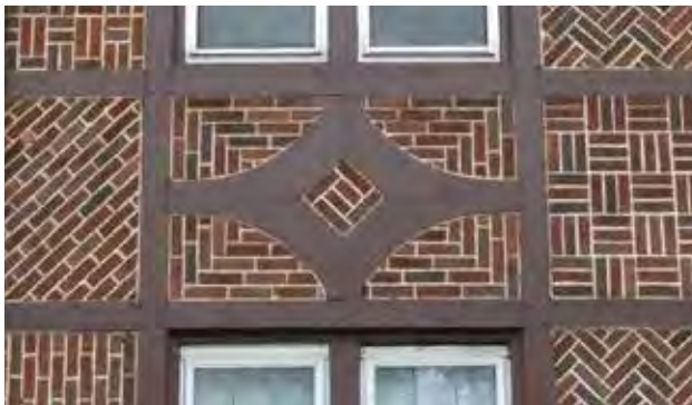
Fig B.3.D.1.e and p: An example of ornamental brickwork in a mixed-use building.
