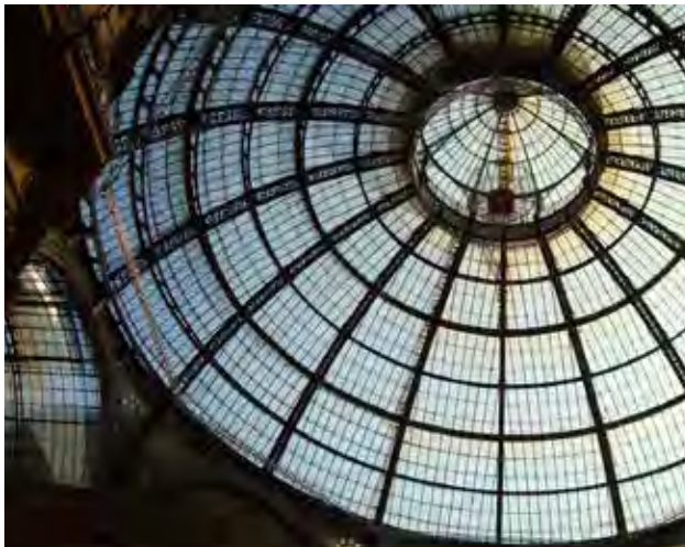
Fig C.1.D.4.b.iv: A skylight is the primary means of illumination in the center of this pedestrian mall.
