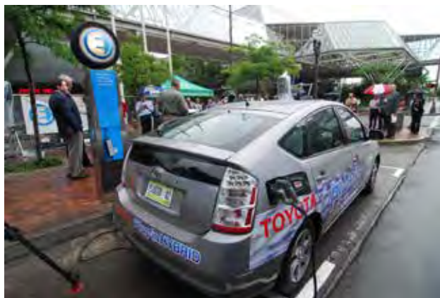
Fig C.1.D.4.b.v: An electric vehicle charging station located in a highly visible place encourages its use.
