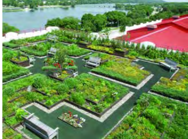
Fig C.1.C.2(2): A modular vegetated roof system reduces stormwater and insulates the roof surface.
