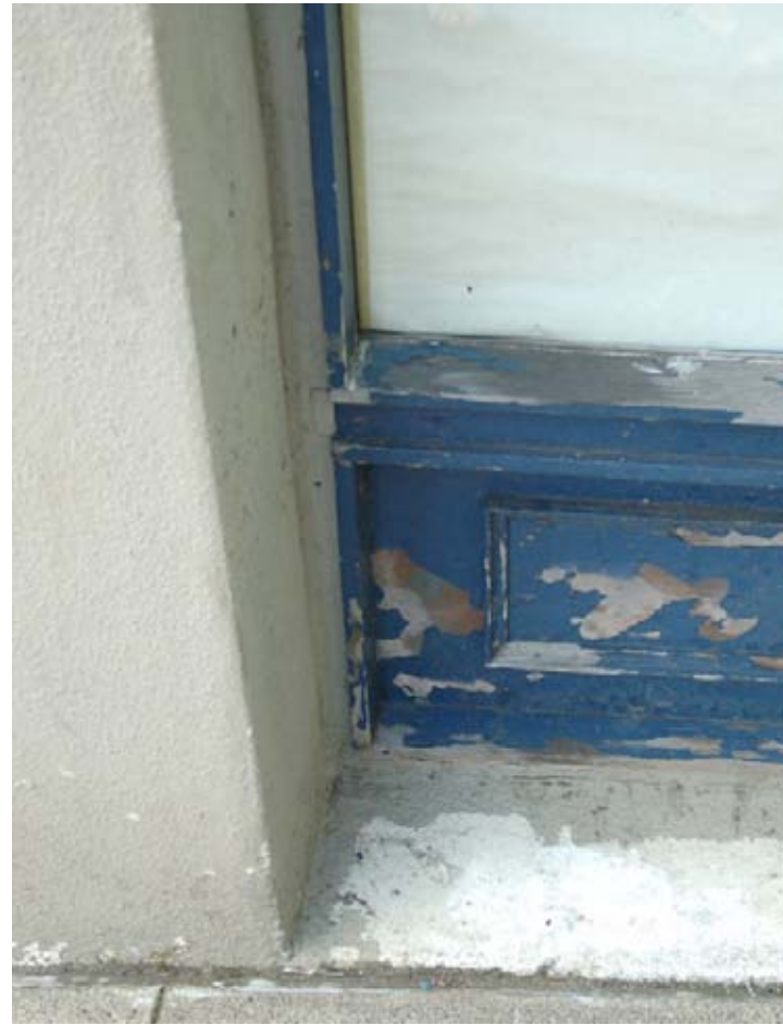
Base in need of paint
