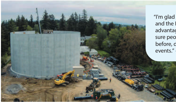
Reservoir construction at the Rockwood Water People's Utility District for the City's joint Cascade Groundwater Alliance project.
