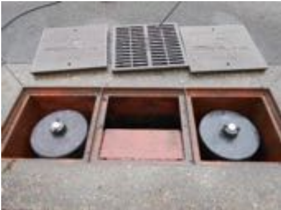
Stormwater filter vault with grate and two filter cartridges, open for cleaning.
