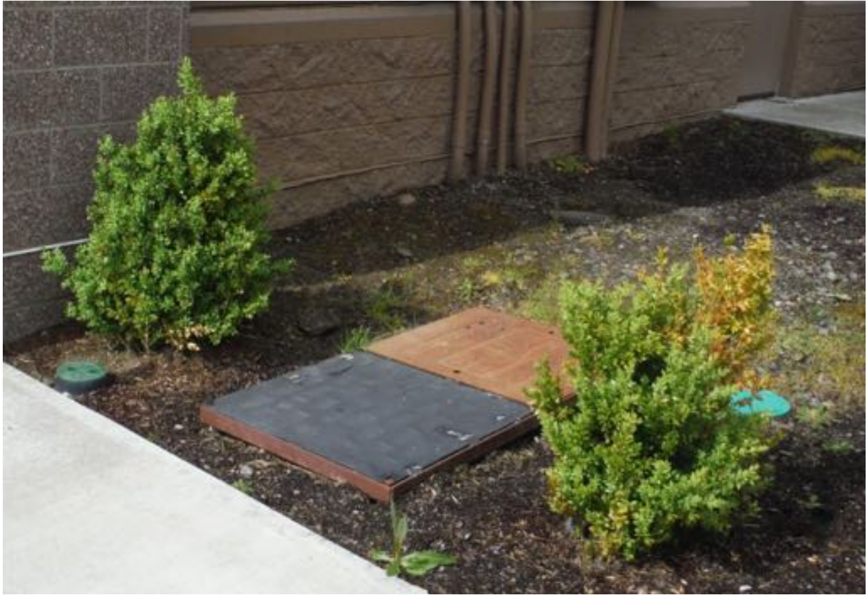
Example photo of a stormwater filter vault. The vaults on your property may be larger or smaller and may be located in a paved area. The metal plates are typically labeled “Contech” or “Stormwater Management, Inc”.
