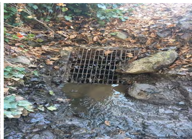
Debris accumulation at outfall located at 6th and Linden Ave.
