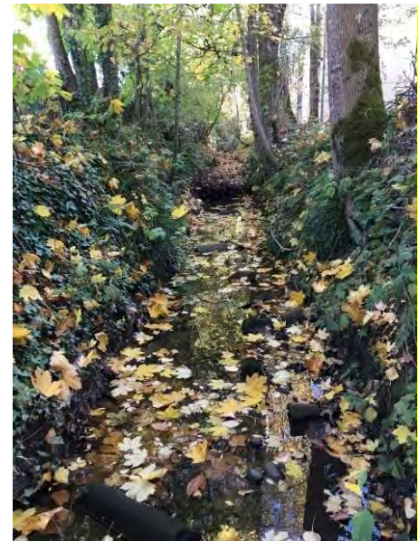
Open channel behind businesses on Division Street
