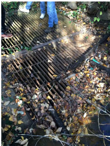
Inlet grate at transition from open channel to pipe section at Chang’s Mongolian Grill.
