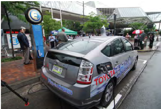
Fig B.4.S3.e: An electric vehicle charging station located in a highly visible place encourages its use.
