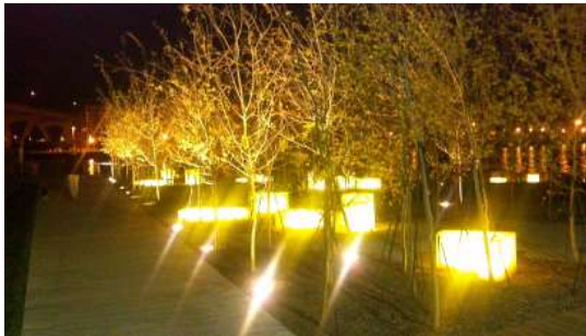
Fig. A.7.G1.c: Light fixtures on the ground prevent landscaping elements from blocking light and creating dark spots.
