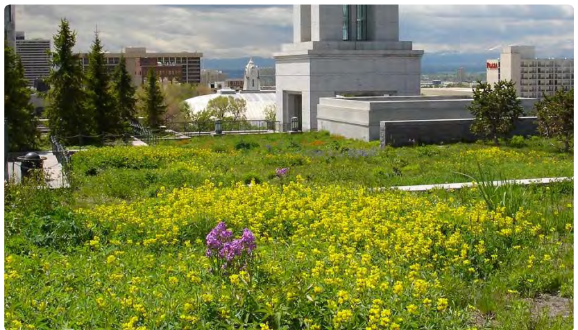
Fig A.6.G3.c: This green roof provides an attractive, sustainable habitat for wildlife.
