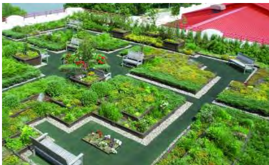
Fig A.6.G3.a: A modular vegetated roof system reduces stormwater and insulates the roof surface.
