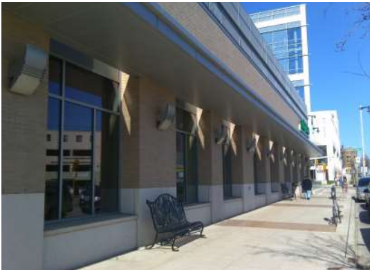
Fig. B.4.S5.c: Projecting sills and wall-mounted lighting fixtures add detail to this commercial building's facade.
