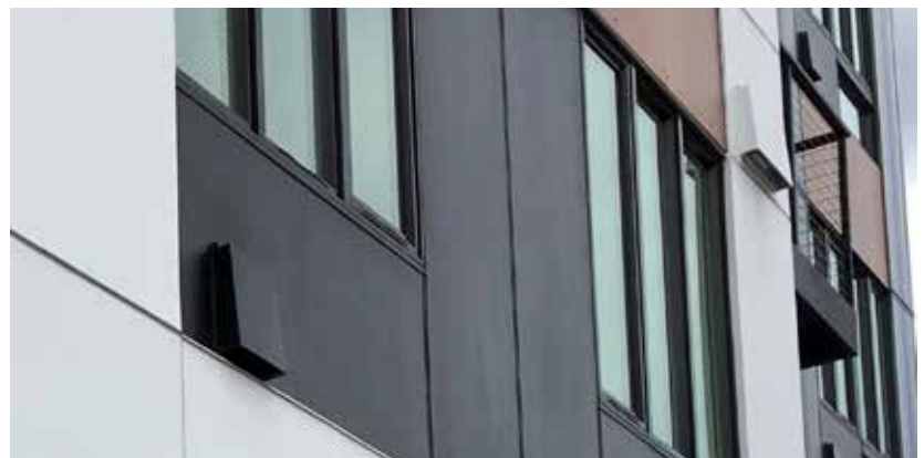
Fig. B.4.S2. Venting on the facade is screened with covers, painted to match the area of the facade they are attached to.
