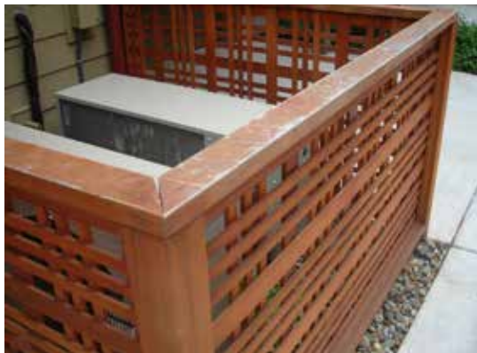
Fig. B.4.S3.a: Ground mounted equipment is screened with a fencing material, consistent with material elements of the primary building.
