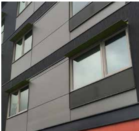
Fig. B.5.S8: Windows on multifamily buildings are recessed a minimum of 2 inches, emphasizing the appearance of depth of the wall.
