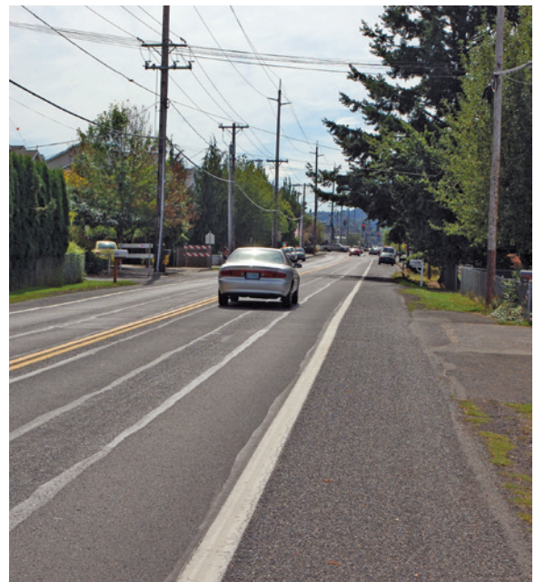
Missing sidewalk along NE Cleveland Avenue north of Burnside Road.
