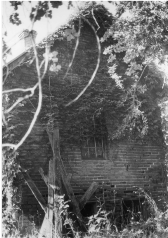
Photograph showing the condition of the buttery building from the natural register nomination (1985)
