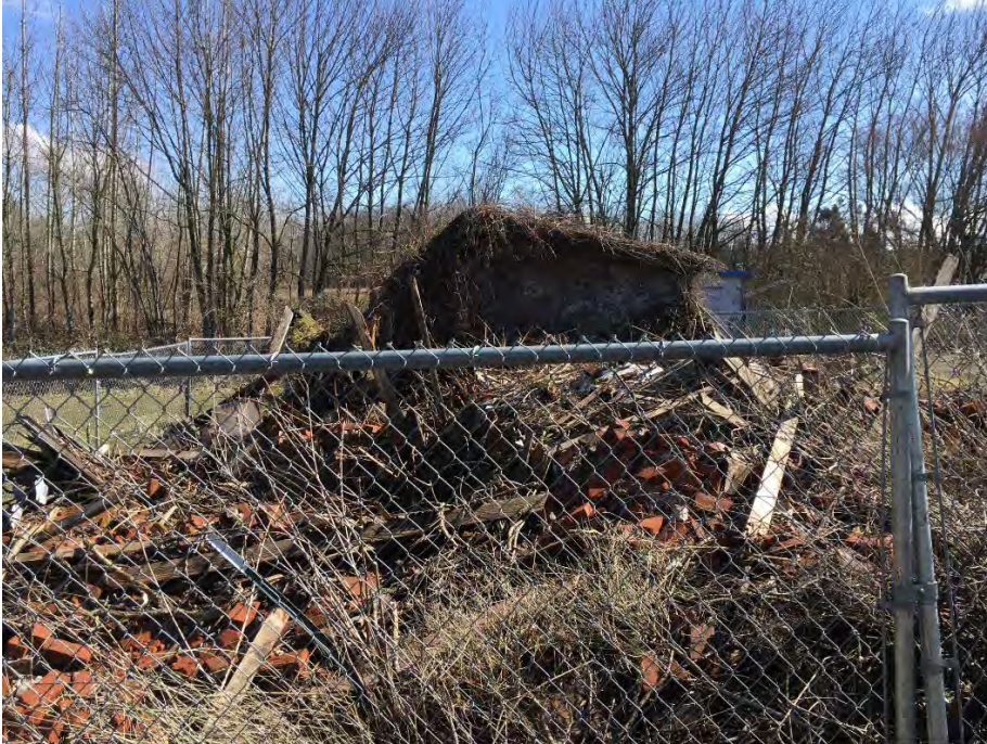
Photo of collapsed garage next to where the Buttery stood, March 2019. In the foreground of the photo, the pile of bricks and debris are the remains of the Buttery.
