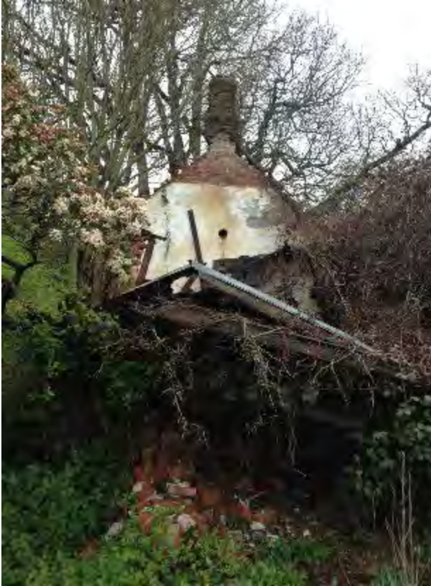
Above photo of the Buttery, April 2016 after it initially collapsed.
